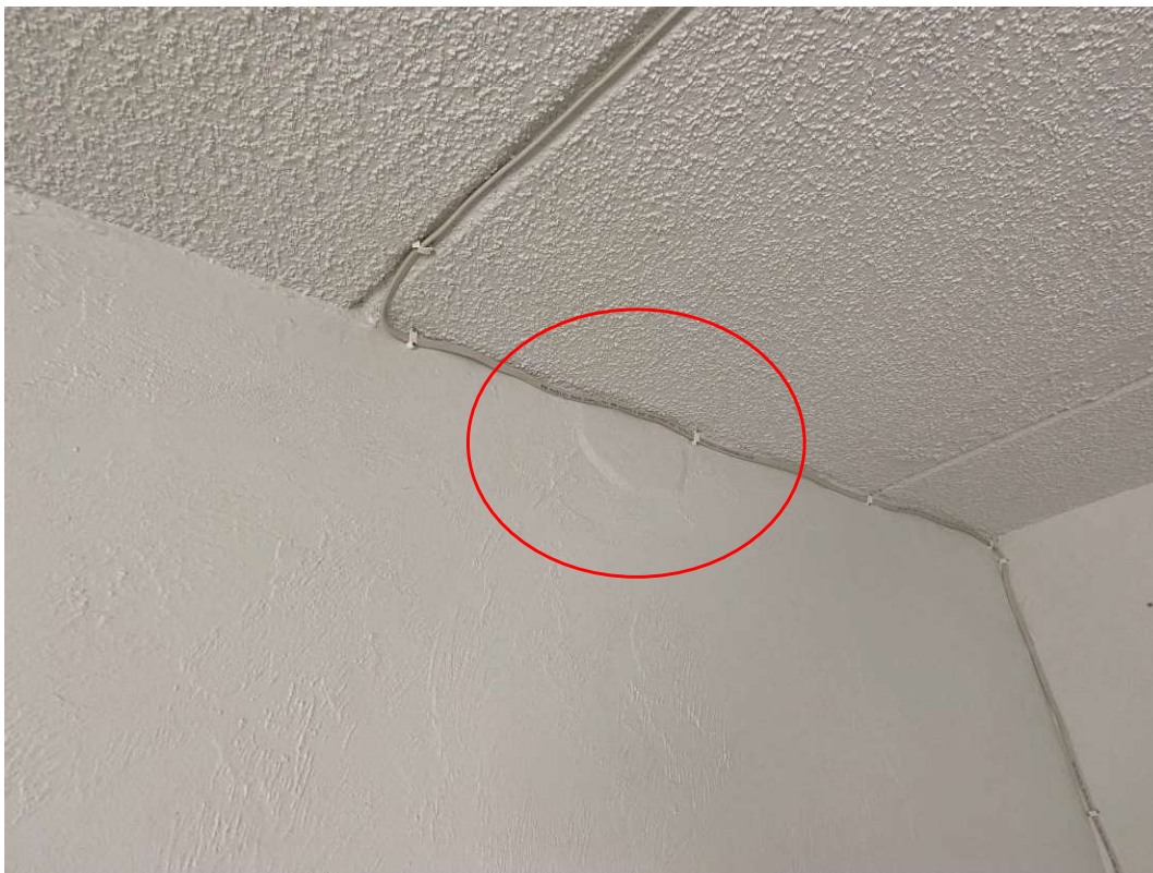
Photograph #2: Bedroom concrete spall in Unit 4
