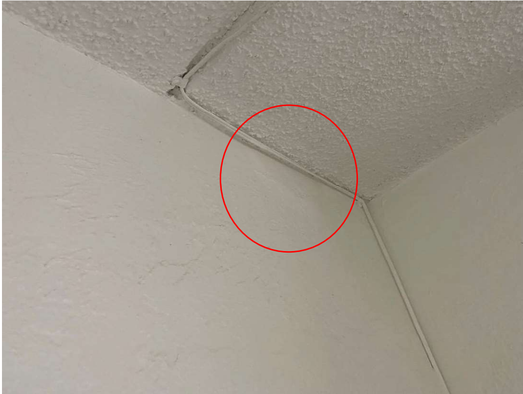
Photograph #3: Living room concrete spall in Unit 4
